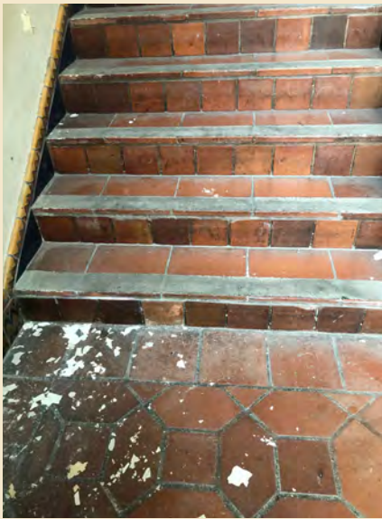
Figure 7.14 The tile mortar at the east stairwell appears to have absorbed water over time as well.
