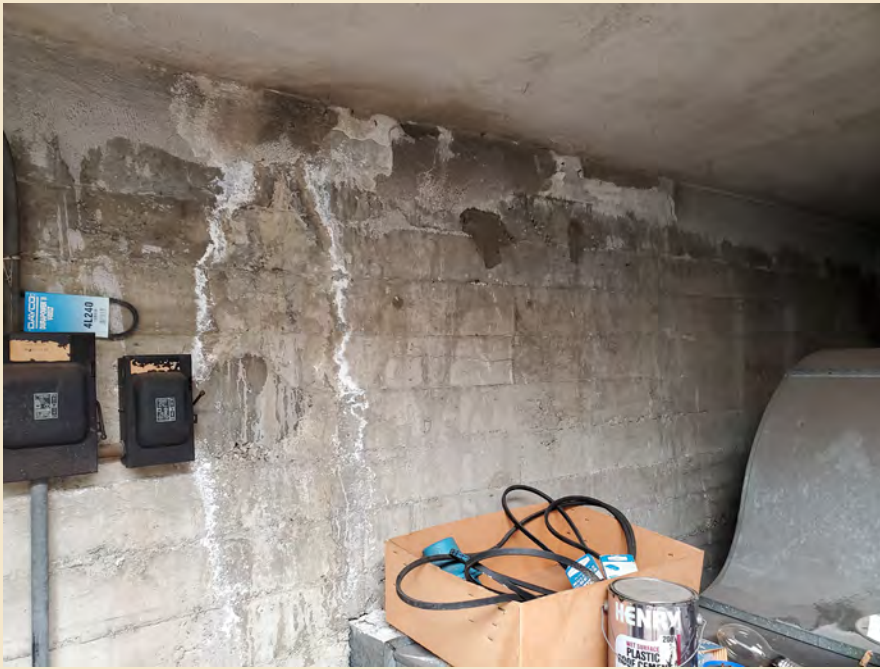
Figure 7.39 The buildup of efflorescence and staining at the north wall of the front attic is indicative of water issues in the roof above.
