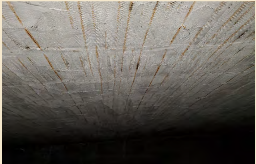
Figure 7.22 Rusting lath is plainly visible through the plaster in the fly loft above the stage.
