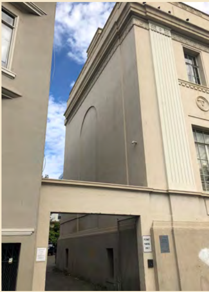
Figure 6.7 The west wing's west elevation is unornamented with the exception of a two-story, semicircular blind arch.
