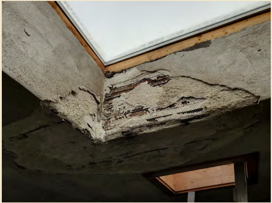
Figure 7.38 The original skylight in the southern roof of the building was replaced at some time (seen here from the attic). The new skylight may be leaking.
