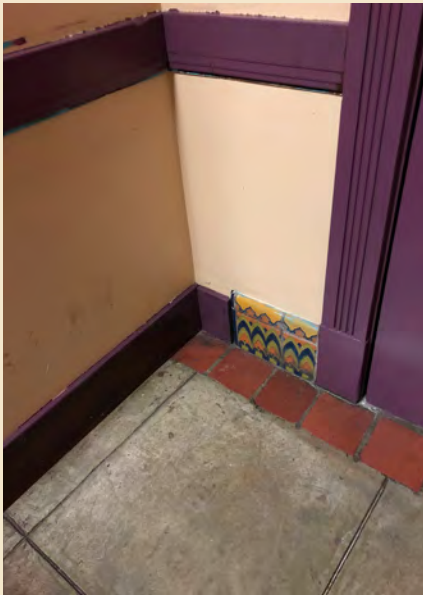
Figure 6.26 Remnants of tile flooring in basement stair landing.
