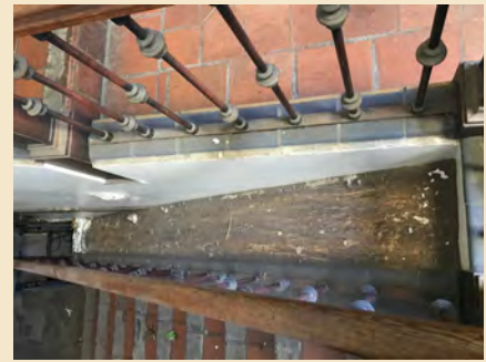
Figure 7.16 At the basement level of the west staircase, a mysterious brown coating has accumulated on the stair carriage between balustrades.
