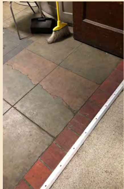
Figure 7.9 Concrete at the west basement stair vestibule is treated inconsistently and is highly worn.
