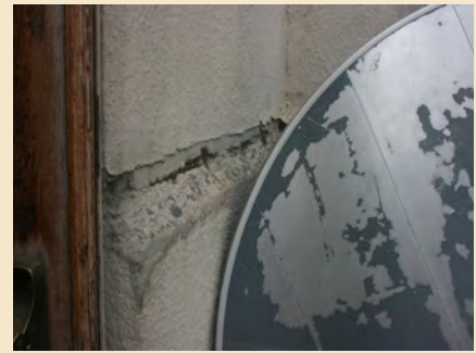
Figure 7.5 At the east courtyard the top of the concrete stem wall has consistently begun to spall, as seen here at the most severe example.
