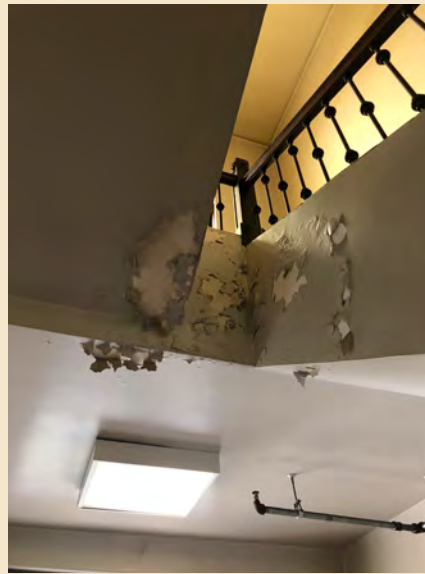
Figure 7.15 Peeling paint on the concrete stair carriage of the west staircase is likely caused by water intrusion.
