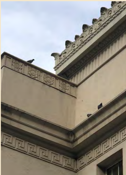
Figure 6.2 The parapet of the center section is taller than the wings and includes bands of fluted, sawtooth, pellet, and nebule molding topped by a row of Acanthus leaves.
