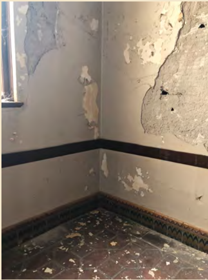
Figure 7.13 Spalling plaster, rusting lath and deteriorated wood wall framing indicate extensive water intrusion at the east stairwell.
