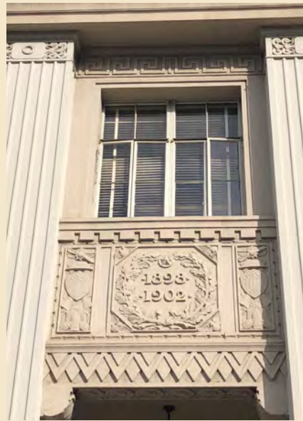
Figure 6.5 Paired two-light steel casement windows with two-light transoms on the second floor.
