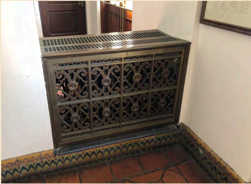
Figure 6.15 Radiators with protective, decorative metal grilles.
