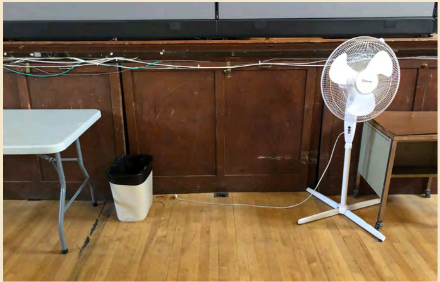
Figure 7.21 The wood stage apron doors do not function appropriately and have significant impact damage.
