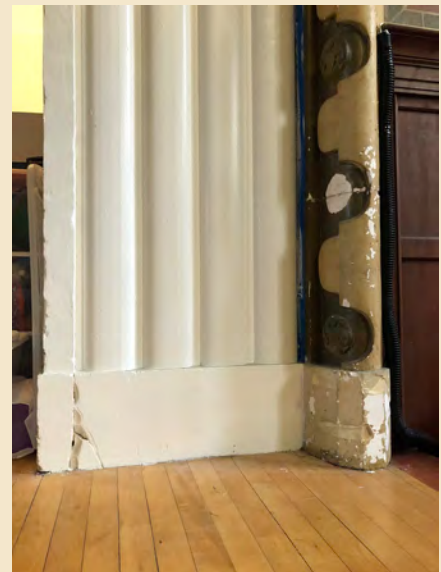
Figure 7.20 The decorative plaster stage proscenium was not originally painted white. A plaster medallion is missing and the plaster is missing and cracked in places.
