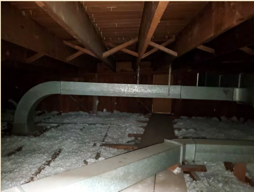
Figure 7.40 The attic over the main corridor and auditorium appear to be weather tight in their current state.
