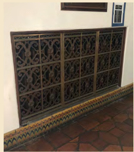
Figure 7.12 The brass decorative radiator grilles are original to the building.
