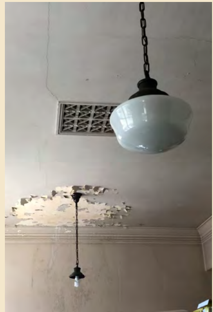
Figure 7.34 A skylight in the attic directly above the dining room ceiling may be the cause of the failing paint seen here at the ceiling.
