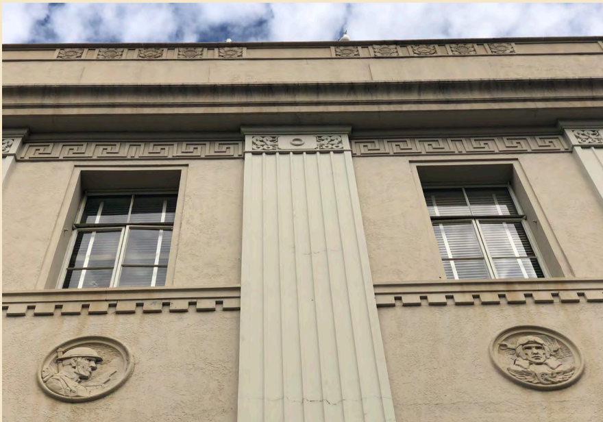
Figure 7.4 Rust staining and consistent cracking along the east façade may be indicative of water intrusion and warrants further investigation.
